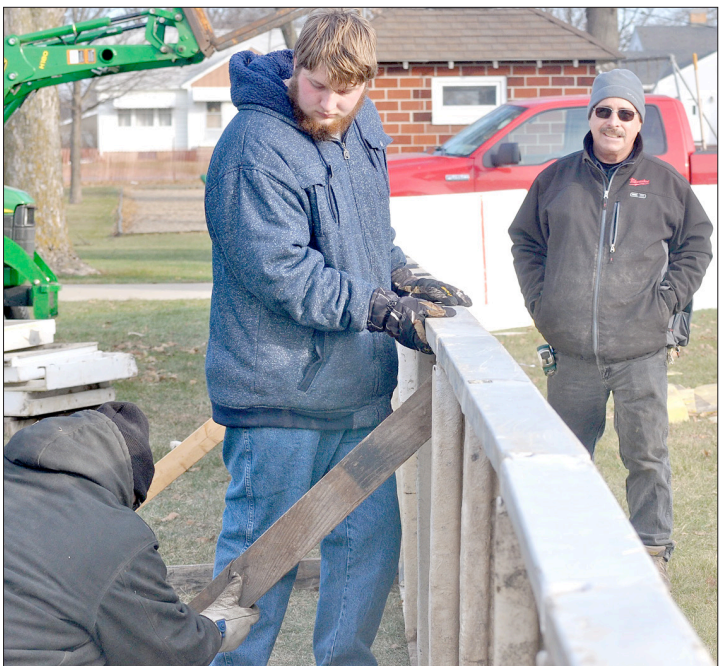
From left to right, John Murray, Dillan Barker and Shane Metz work on the new ice rink at the Dike City Park. The project cost around $1,000 and should be completed in the next few weeks. (Robert Maharry/The Grundy Register photo)
